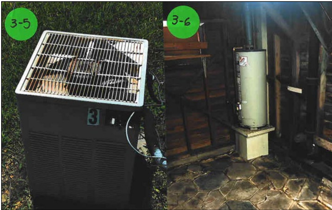
Figure 6: Outdated mechanical equipment to be upgraded to meet code
