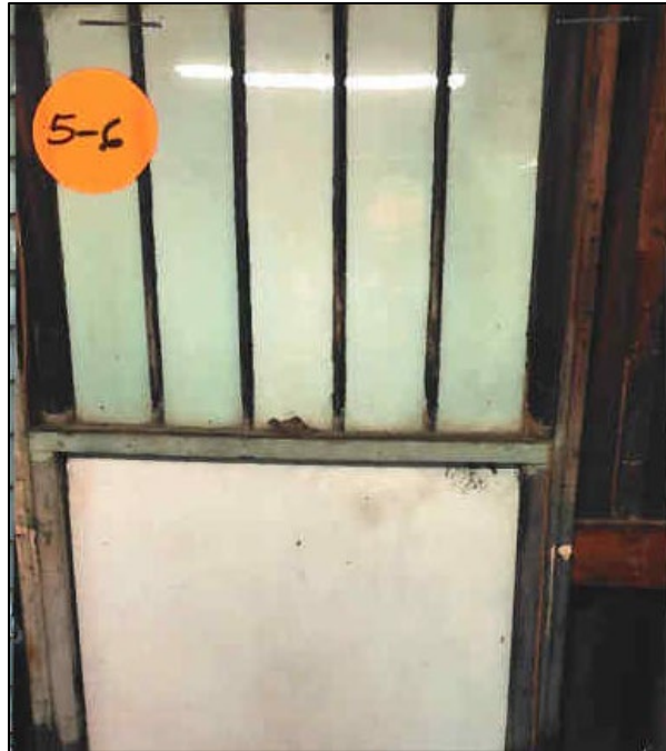
Figure 7: Window to be replaced with new impact window to replicate configuration Appendix B: Post-Construction Photographs (2022)
