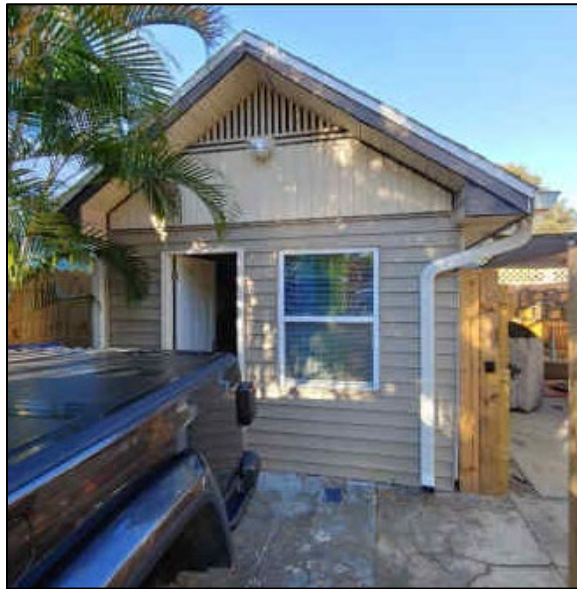
Figure 1: Front façade of garage building. Garage door had been removed and inappropriate door and window were installed.
